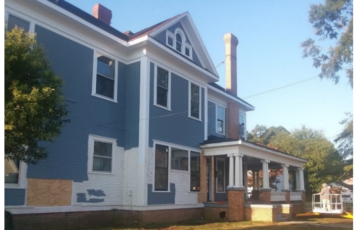
The House of Hope in Kinston, North Carolina, a 16-bed transitional housing facility restored by Hope Restorations, Inc.
